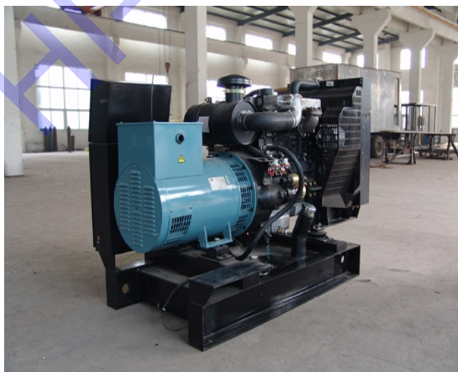
Perkins genset in factory
